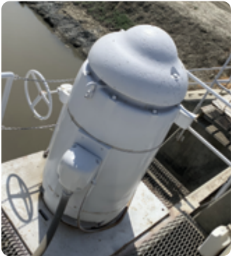
Canal Lift Pumps
